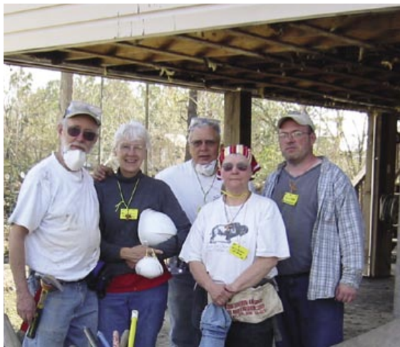
FROM LEFT: John Dutcher, Bonnie Orsini, Larry Orsini, Anita Dutcher, and Fr. David Blake, OFM, under a house they gutted to prep it for restoration. Houses there are on stilts to protect them from flooding -- except that Katrina waters rose to 25 feet, engulfing most everything.
